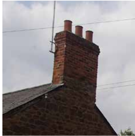
Rectangular brick chimney at edge of ridgeline and central to gable, Bloxham
